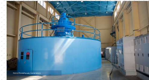
Holm Powerhouse Generators
